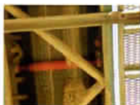
Conveyor belt idler
